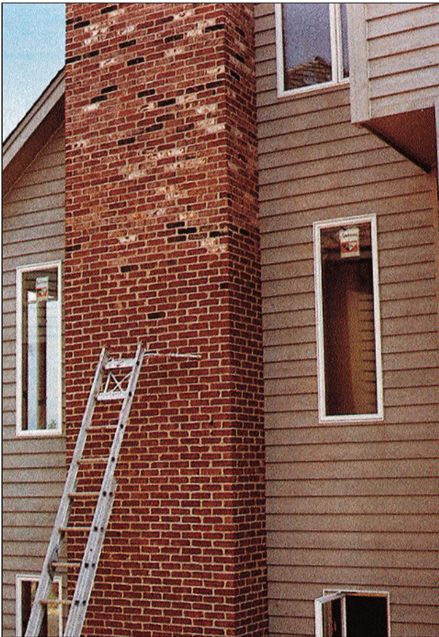
Too few range brick were delivered and installed, resulting in an uneven and unacceptable appearance.
