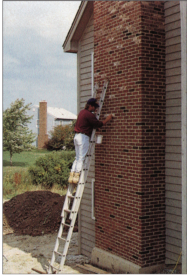
"Masonry artists" apply water-based, multipolymer stain and create the desired color blend.
